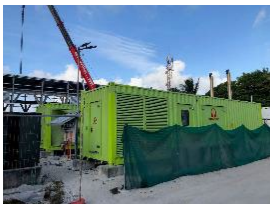
The new Betio powerhouse, constructed by the Public Utilities Board, with NZ-funded generator units in the foreground. Credit: Kiribati Public Utilities Board
