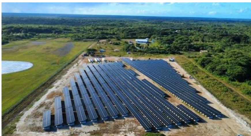
The completed renewable energy site in Niue. Credit: Sunergise
