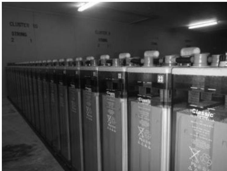
Figure 27: Labelling of clusters, strings and batteries
