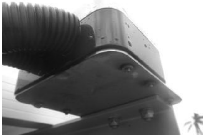
Figure 39: Rusted bolts on SMA sensor module
