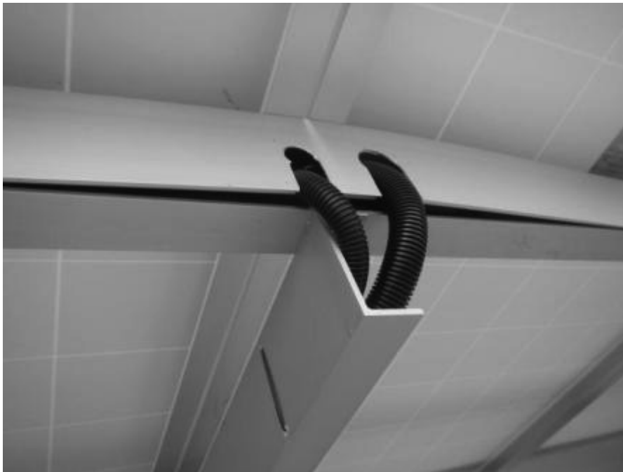
Figure 44 Conduit entry to ducting
