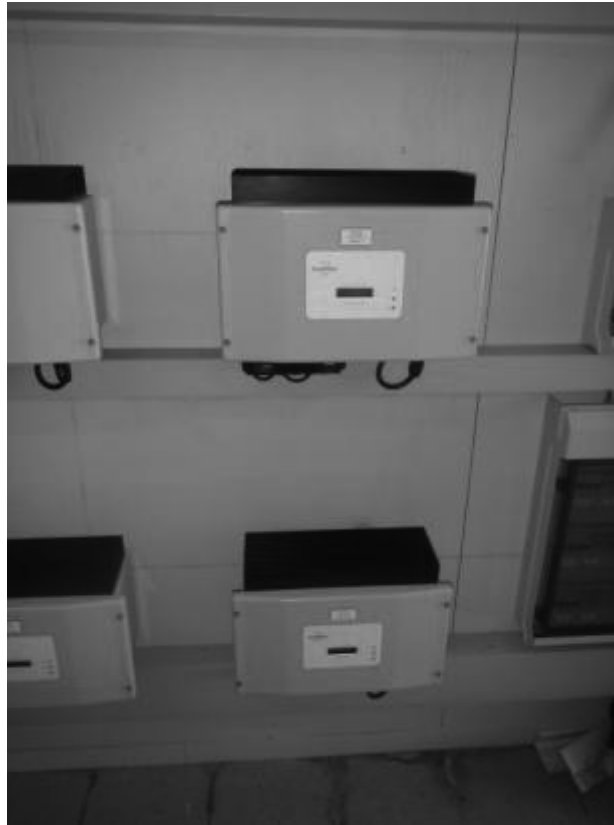
Figure 16: Labelling on inverters
