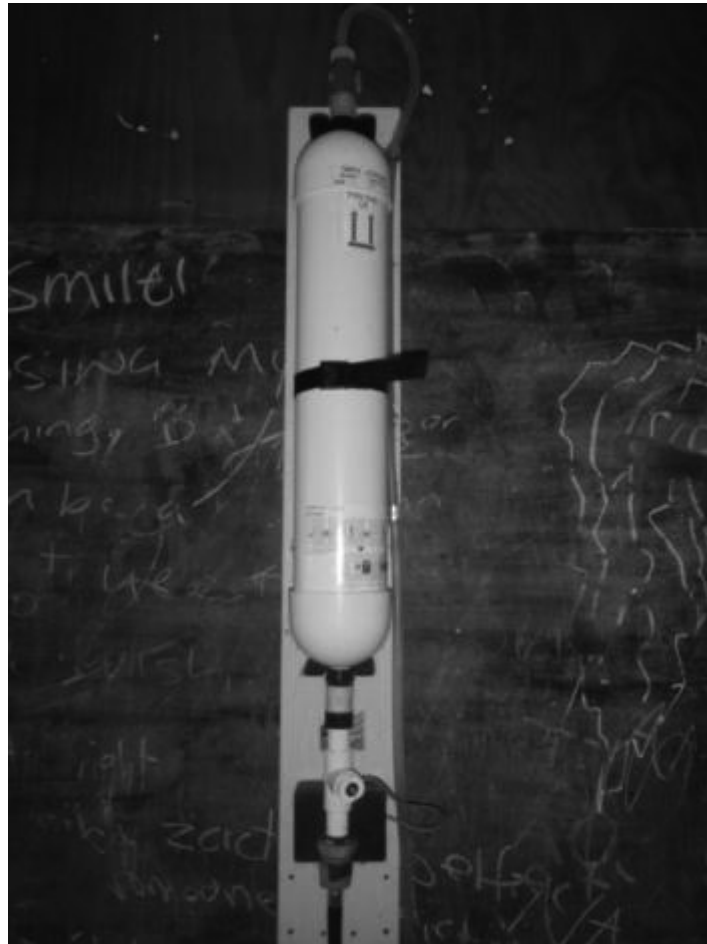
Figure 23: Deionizer mounted on wall in battery room
