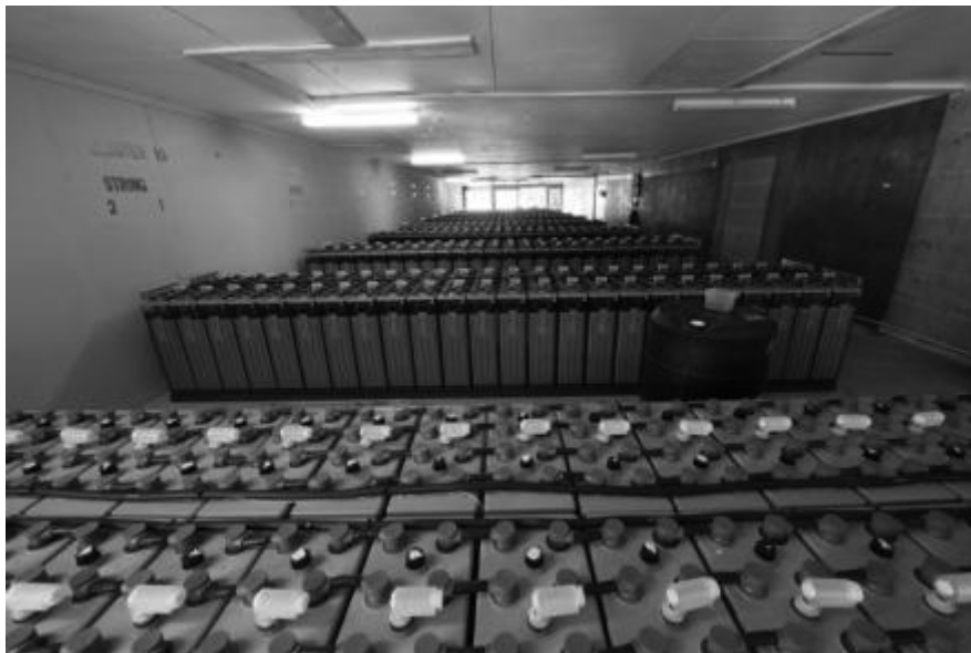
Figure 35 Drum of battery acid next to batteries
