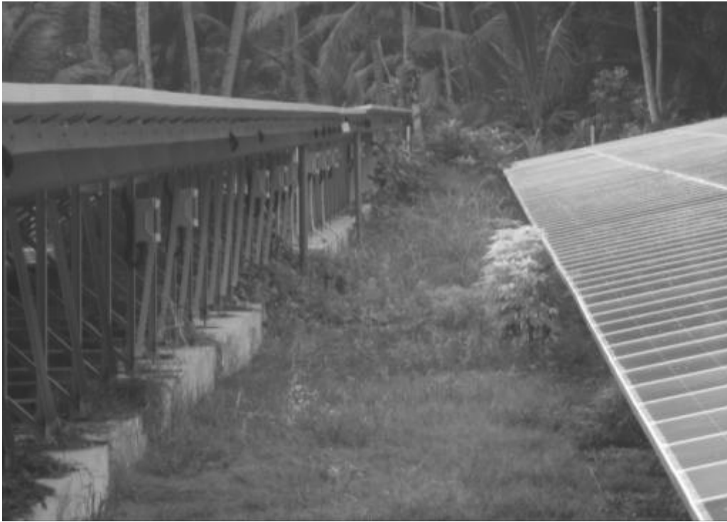
Figure 32: Excessive vegetation around array including plants shading panels and creepers on framing
