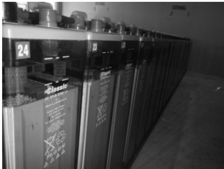
Figure 36: Battery electrolyte levels close to maximum line
