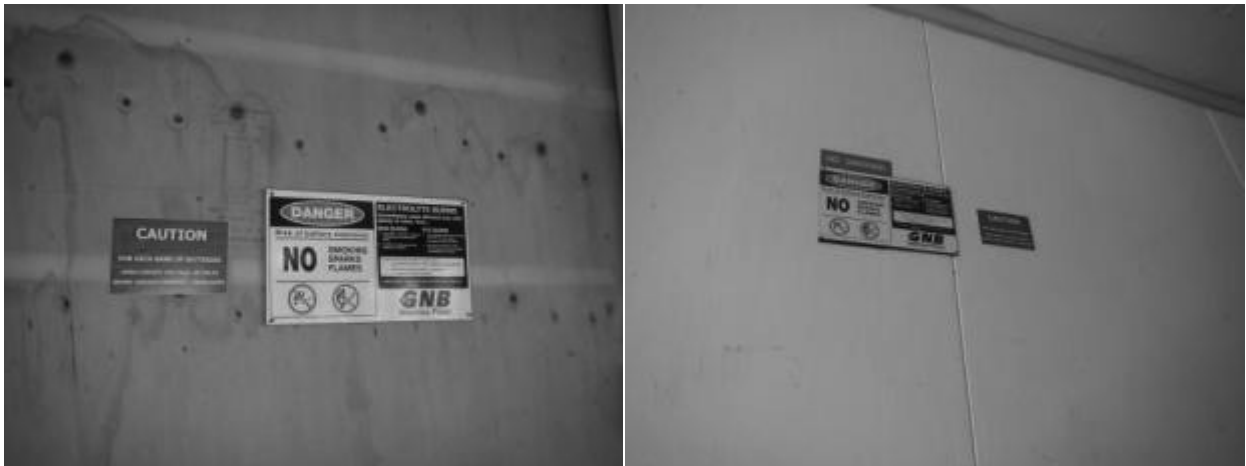
Figure 26: Warning labels at both ends of battery room
