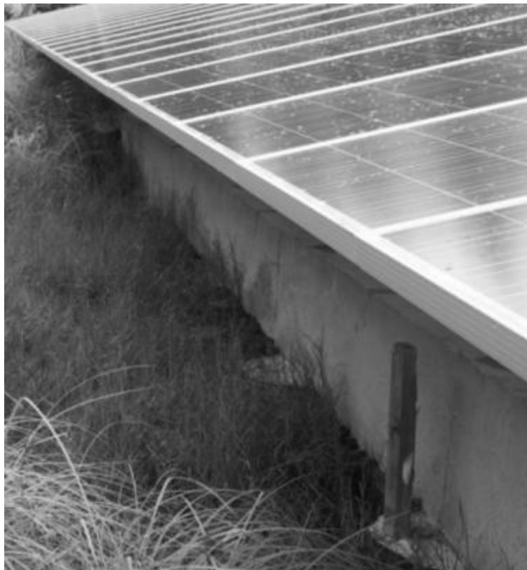
Figure 4: Foundations in swampy ground appear unsupported
