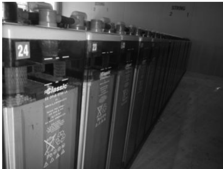
Figure 25: Water level on batteries near maximum line
