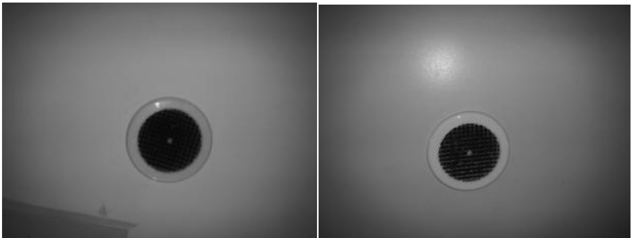
Figure 13: Extractor fans in the centre of the inverter room
