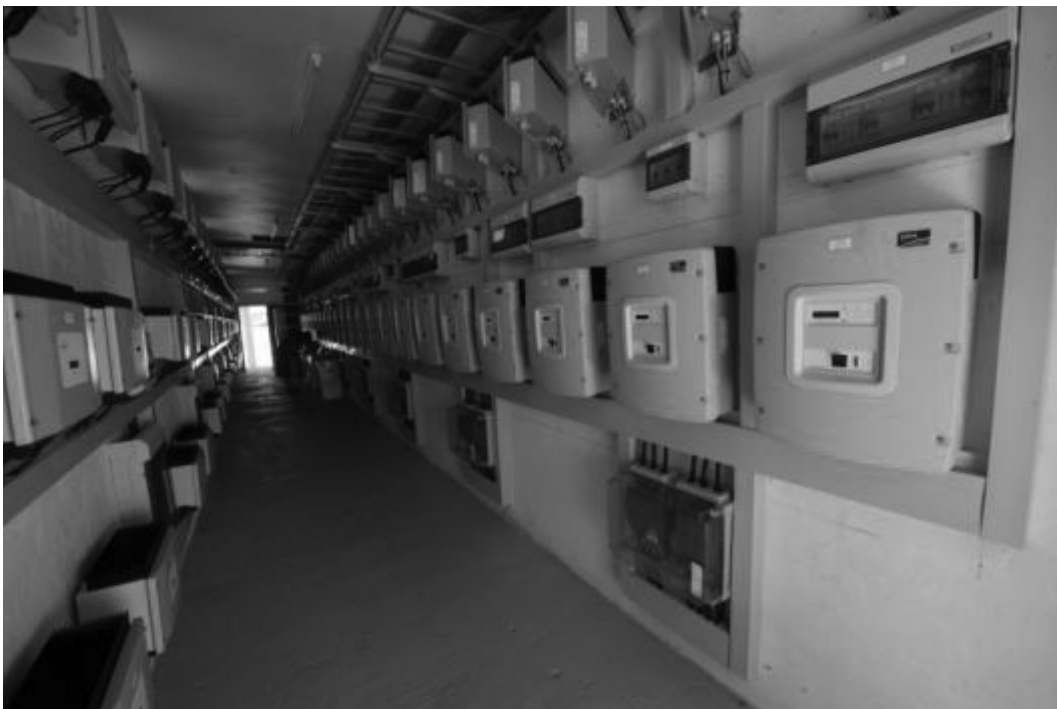
Figure 48: Naturally ventilated inverter room
