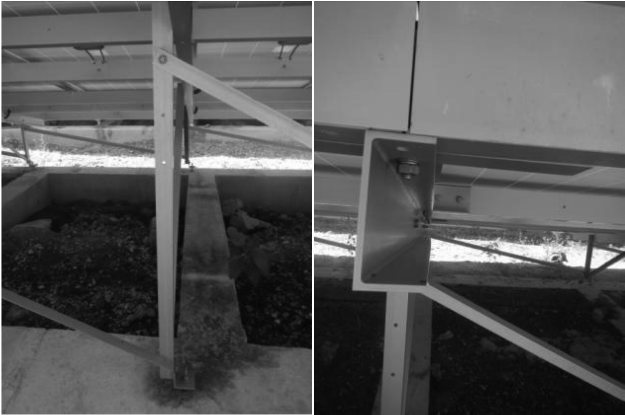
Figure 2: Array frame detail showing general condition of array frame and bolts
