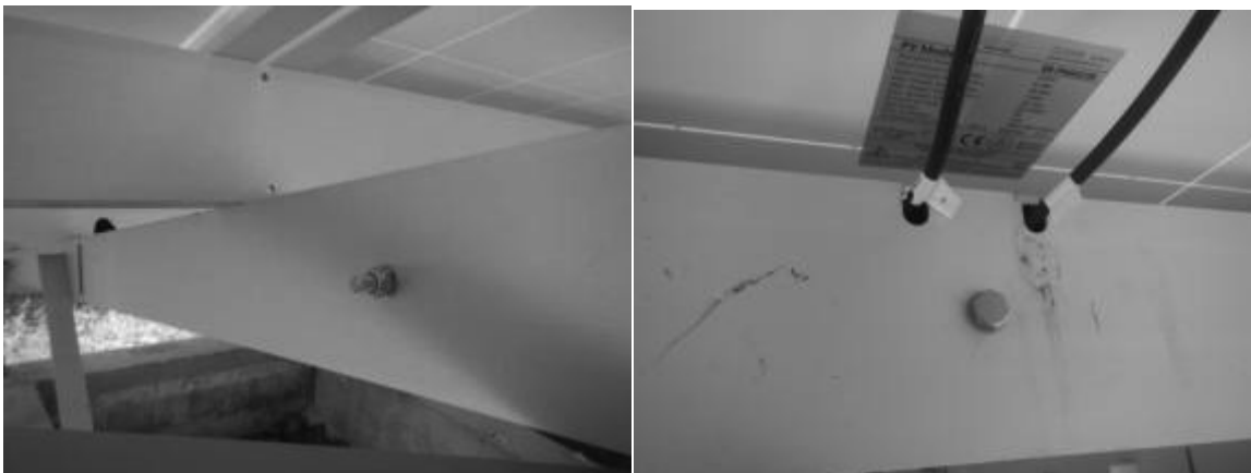
Figure 1: Array frame detail showing typical bolt (left) and residual rust marks from steel strapping (right)
