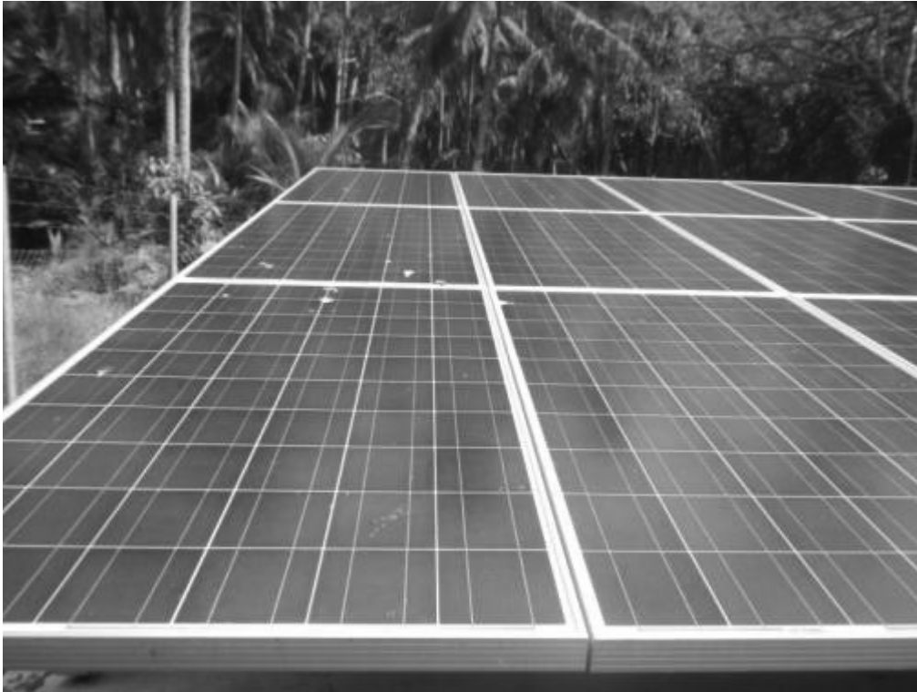
Figure 29: Panels are mostly clean with the exception of some bird droppings
