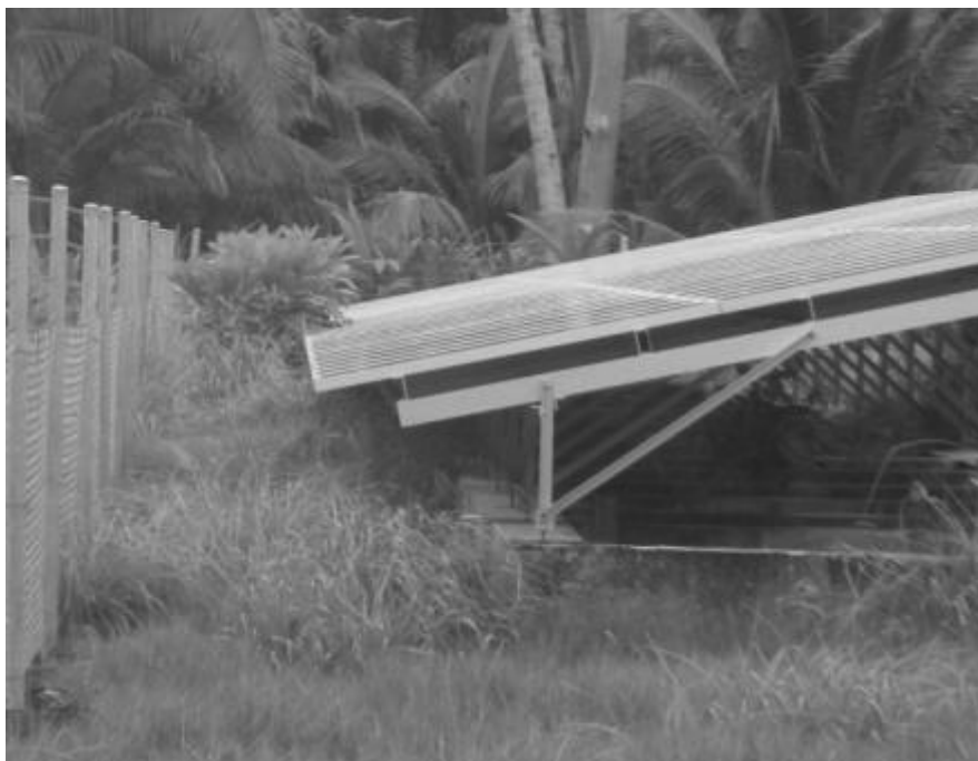
Figure 31: Plant shading the array. Overgrown vegetation in this area makes it difficult to access the eastern end of the array
