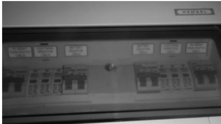
Figure 17: Lightning arrestors flagged green
