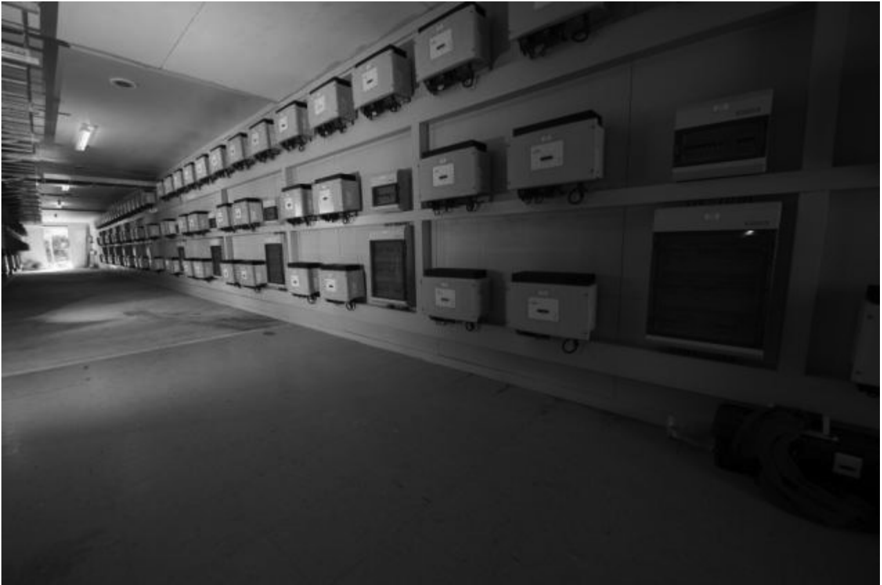
Figure 12: Inverter wall and extractor fans visible in ceiling
