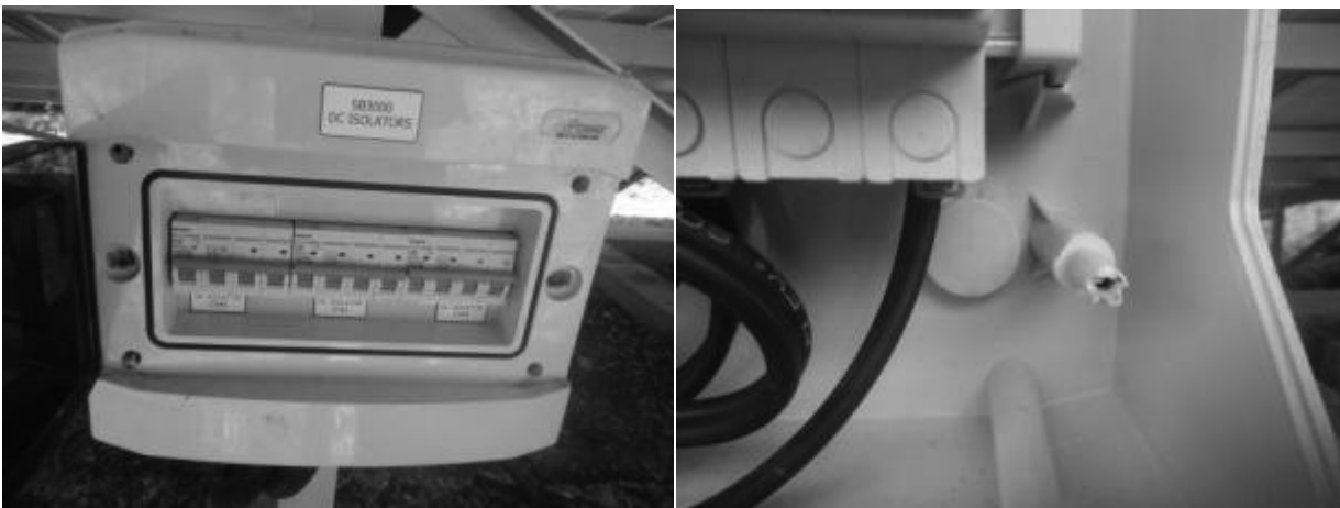
Figure 9: Isolator with damaged screw (left) and signs of wear on screw mounts (right)
