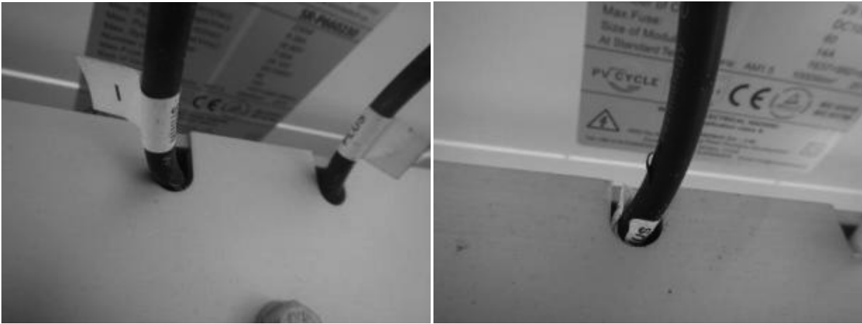
Figure 7: Cable entries to ducting – some scratches visible
