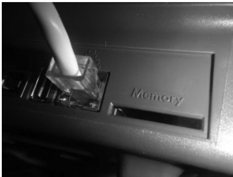
Figure 21: SD cards missing from Webboxes
