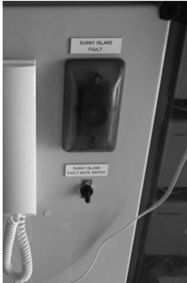
Figure 50: Alarm mute switch in “OFF” position
