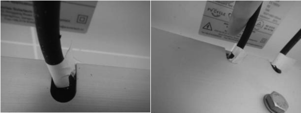
Figure 43: Cable entries to ducting – some scratches visible
