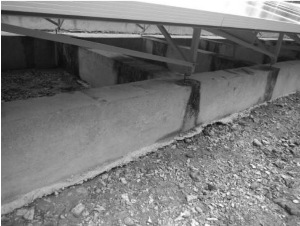
Figure 41: Concrete footings showing some preliminary erosion of soil
