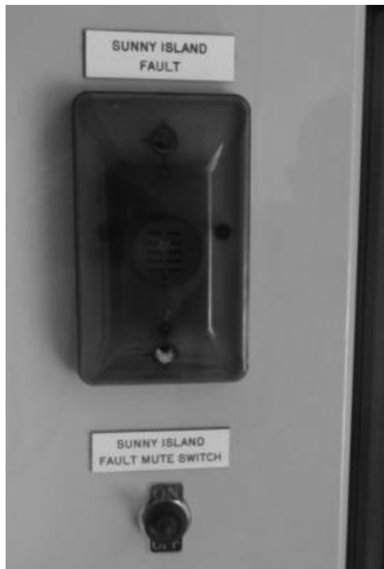
Figure 15: Sunny Island Fault Mute Switch is on
