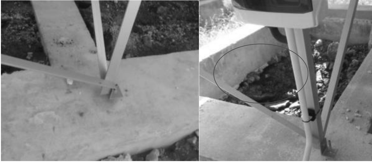
Figure 3: Typical concrete footing detail (left); signs of erosion around foundation (right)
