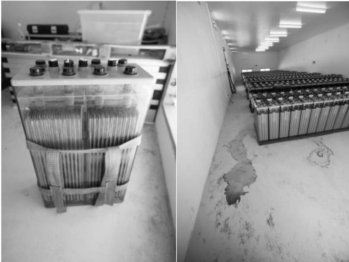
Figure 99: Dead cell, and storage area in battery room (left), water on floor (right)
