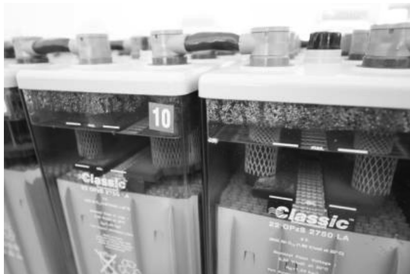
Figure 67: Battery electrolyte levels
