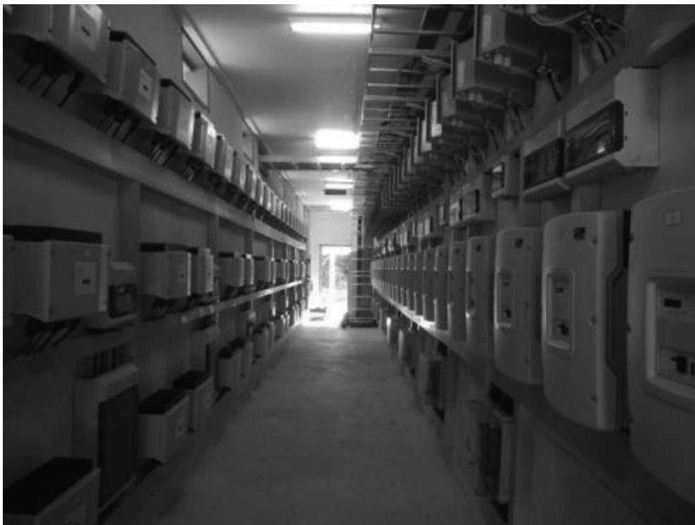
Figure 80: Inverter room with natural ventilation (top left)
