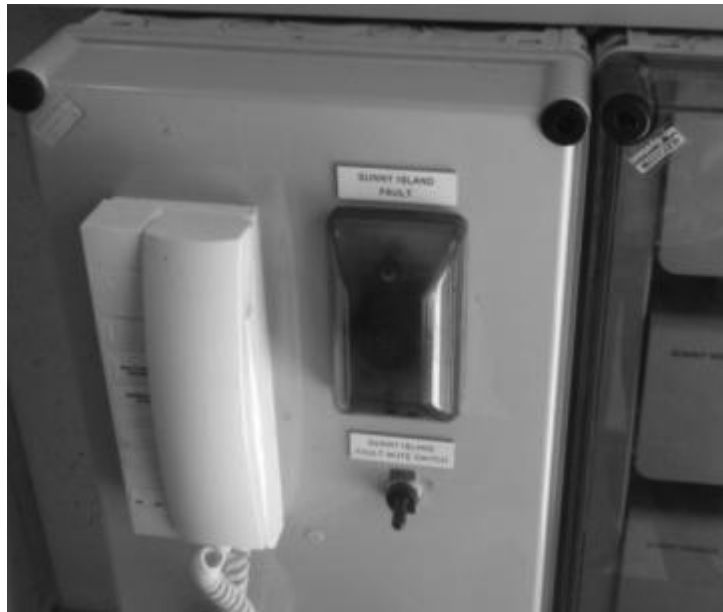
Figure 82: Fault mute switch in OFF position
