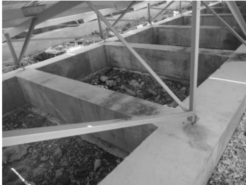
Figure 71: Array frame detail
