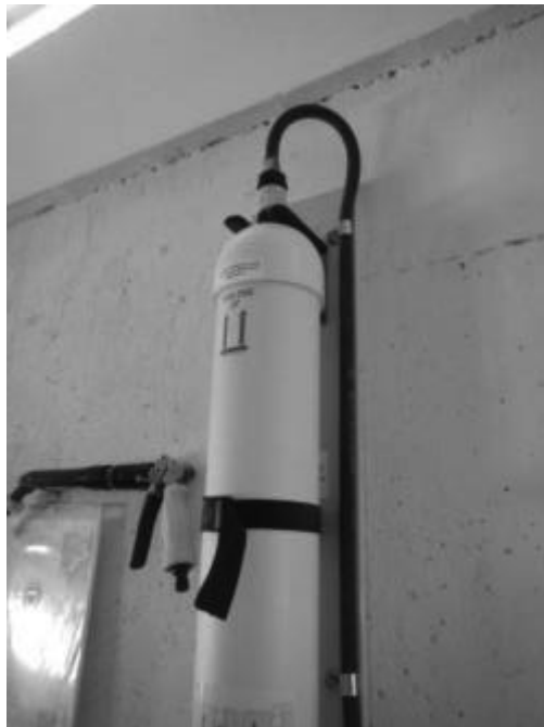
Figure 57: Deionizer in battery room
