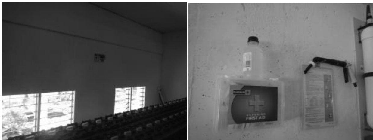
Figure 60: Battery room warning labels
