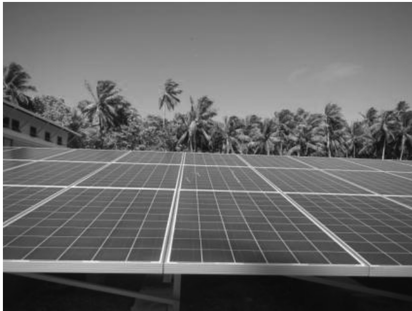
Figure 95: Panels generally clean
