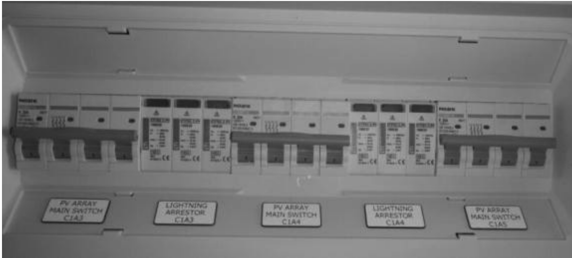
Figure 52: Sunny Boy lightning arrestors intact (red button pops out when tripped)
