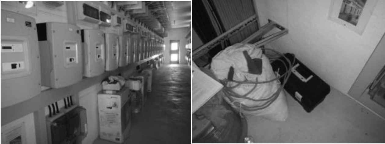
Figure 64: Inverter room, spare Sunny Islands (left), toolbox and miscellaneous items (right)
