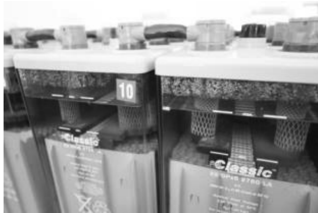
Figure 59: Battery water levels close to maximum line
