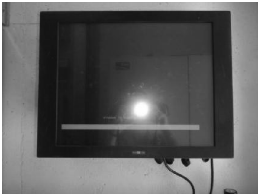
Figure 81: Inverter room computer failed to boot due to hard drive failure
