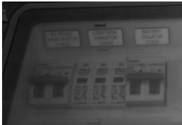
Figure 53: Lightning arrestors flagged green
