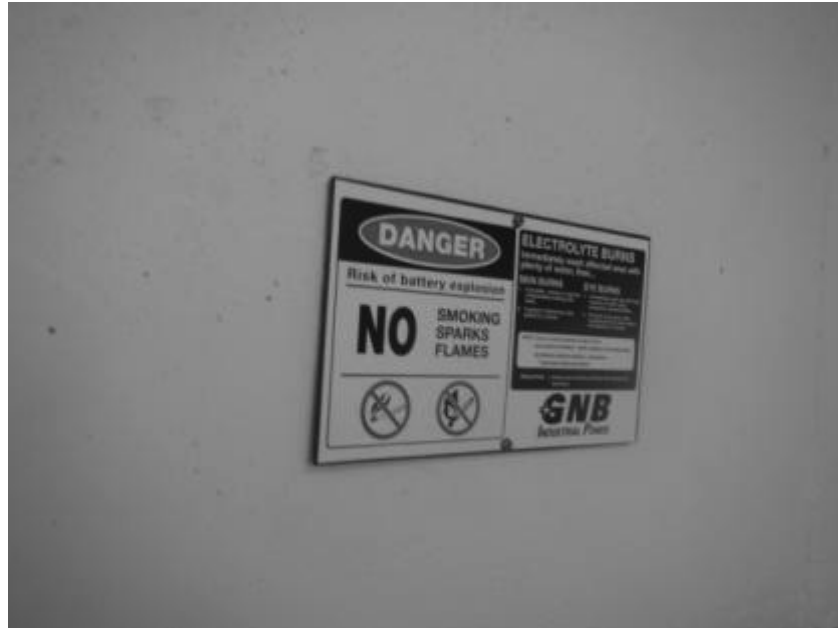
Figure 93: Warning labels in battery room
