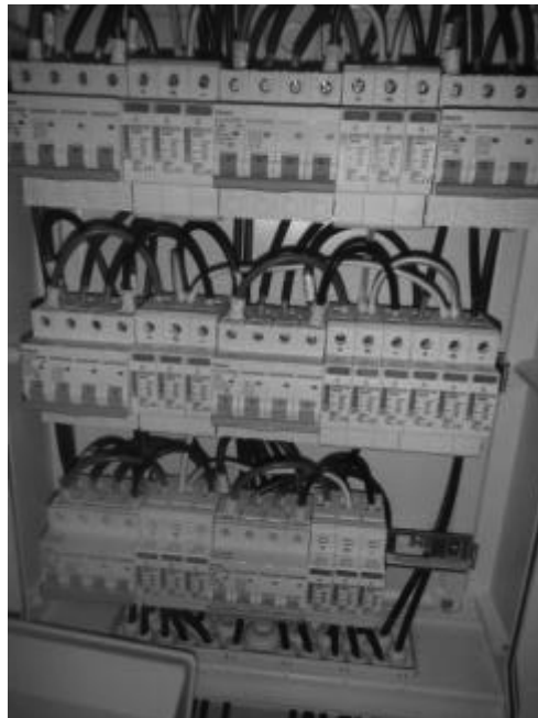
Figure 87: DC isolator wiring
