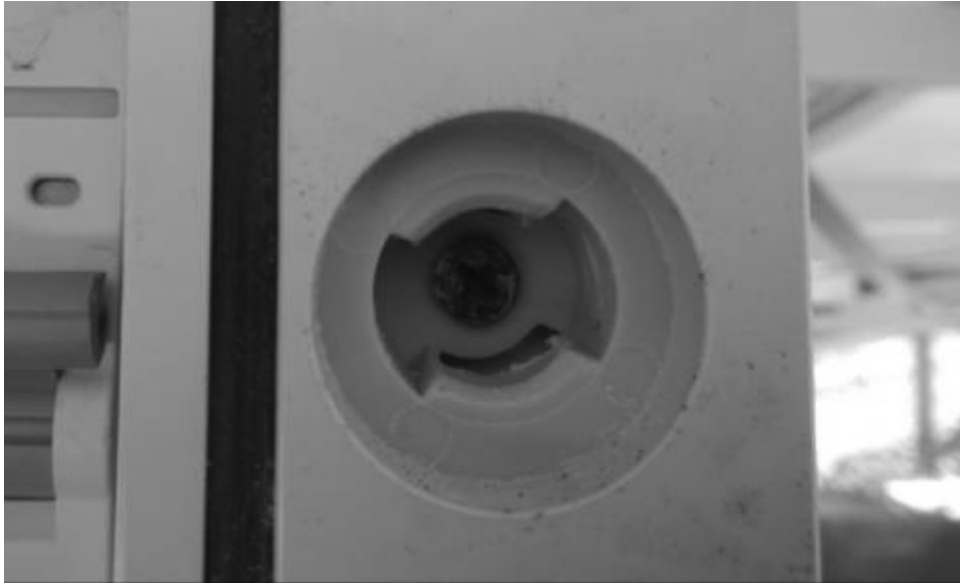
Figure 79: Corroded galvanized steel screw on enclosure latching mechanism
