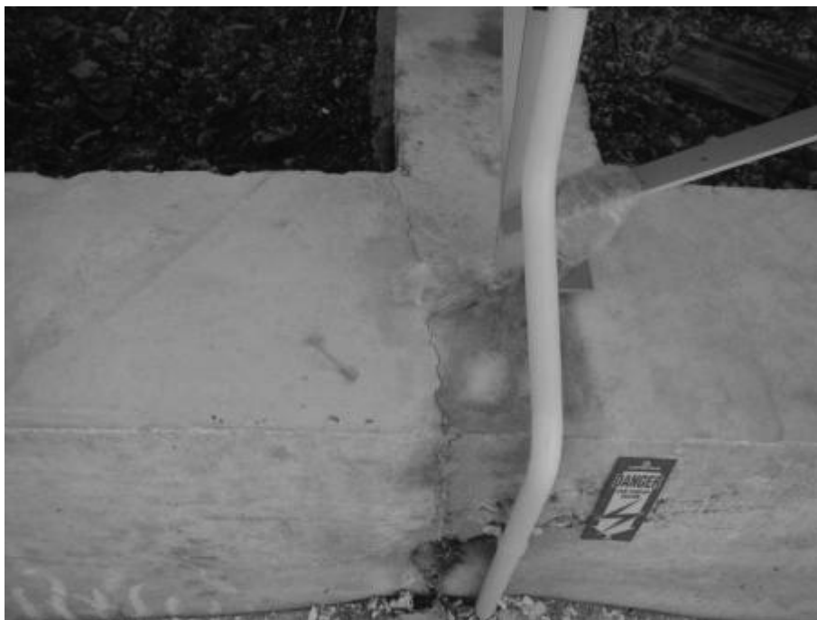
Figure 72: Small cracks in concrete foundations
