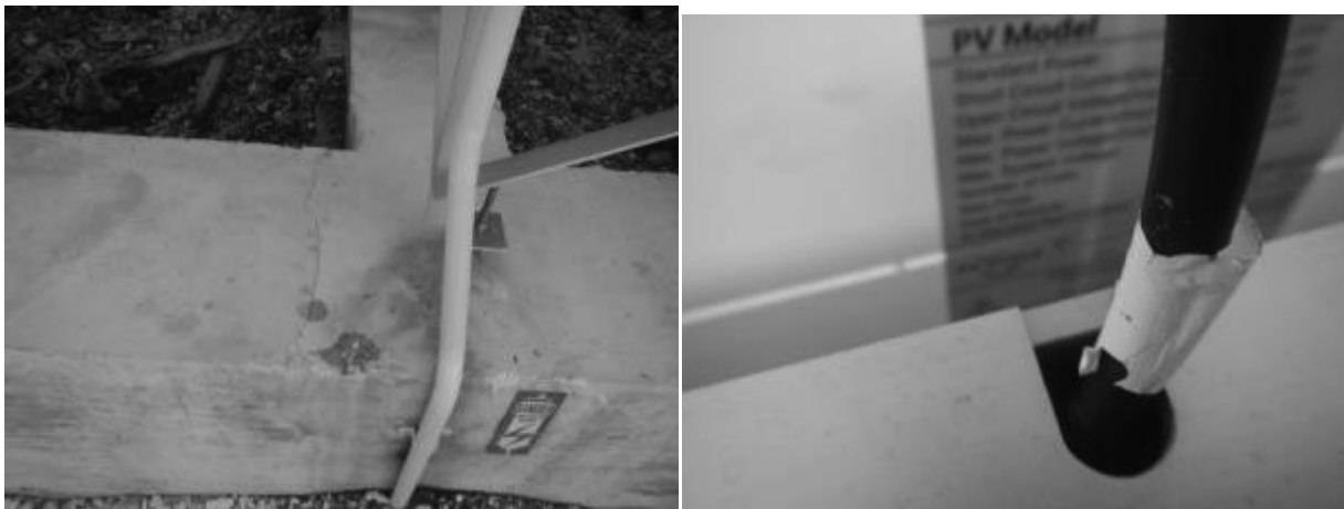
Figure 74: Conduit detail (left) and minor scratches on cables (right)
