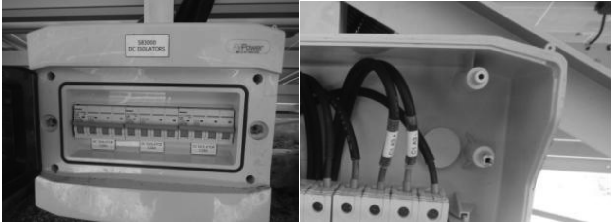
Figure 75: Isolator enclosure labelling (left) and screw mounts (right)
