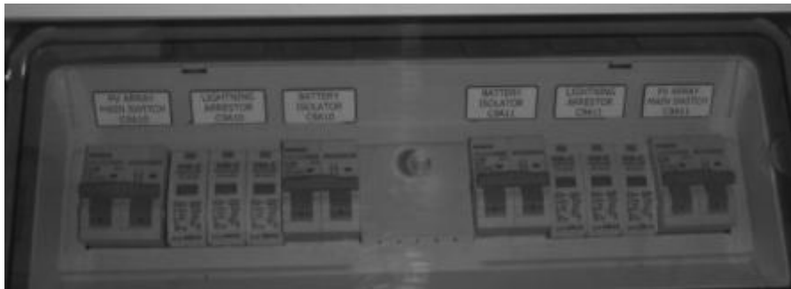
Figure 85: Surge arrestors intact
