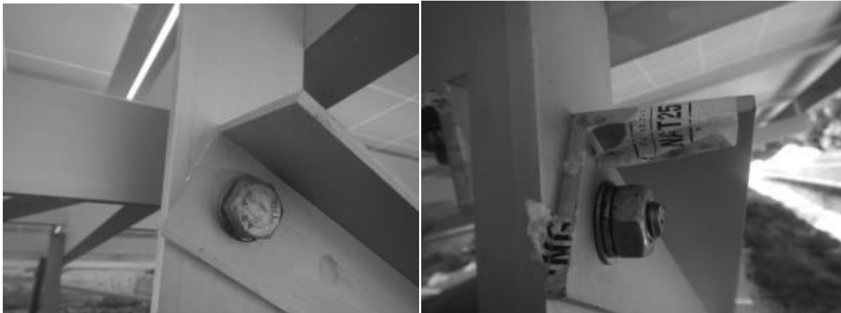
Figure 70: Tea staining on bolts on the array frame
