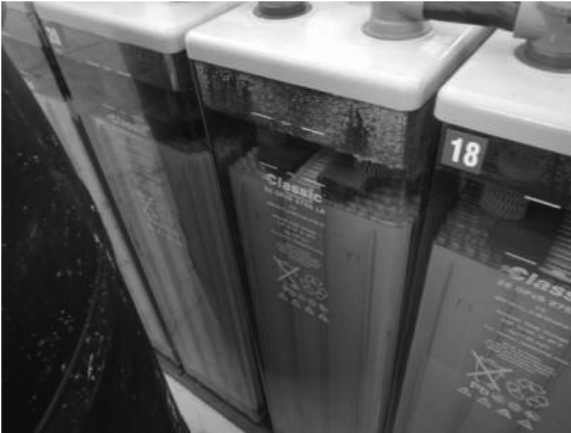
Figure 92: New battery with some orange debris floating in the water
