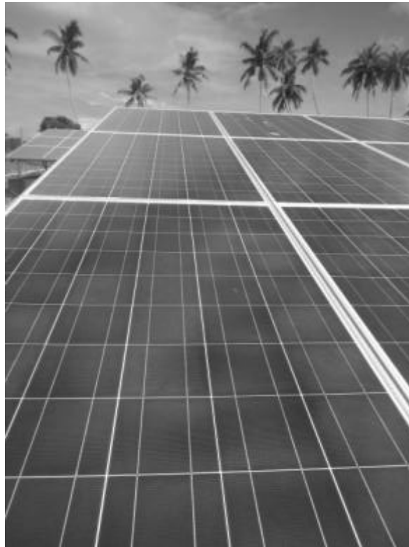
Figure 62: Panels generally clean, some bird droppings at top
