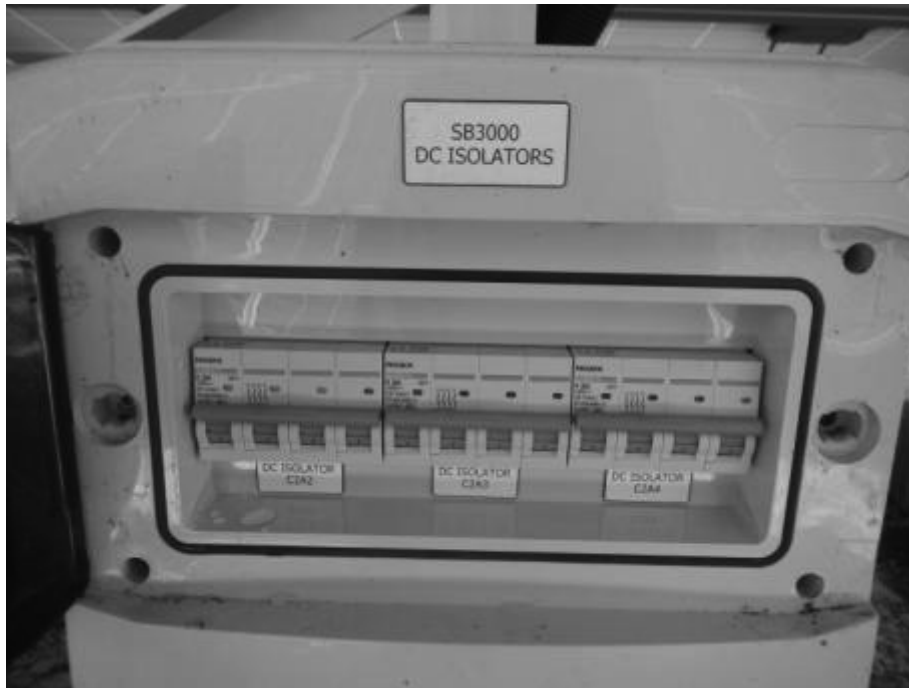
Figure 77: Water and mud on outside of isolator enclosures after a major storm
