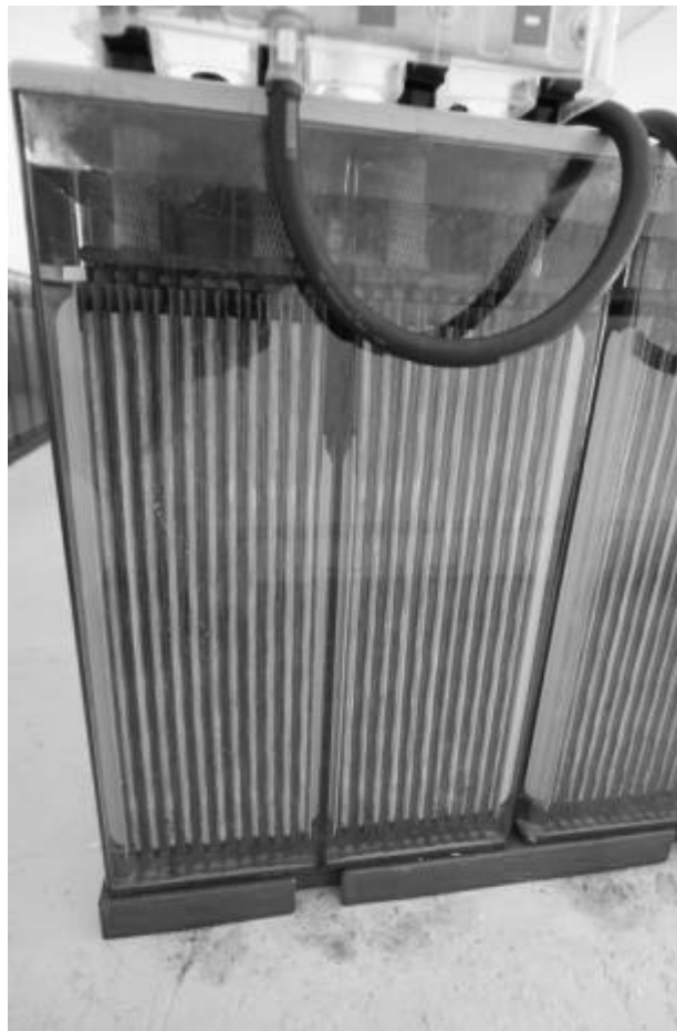
Figure 58: Battery plates and small lead deposits at bottom
