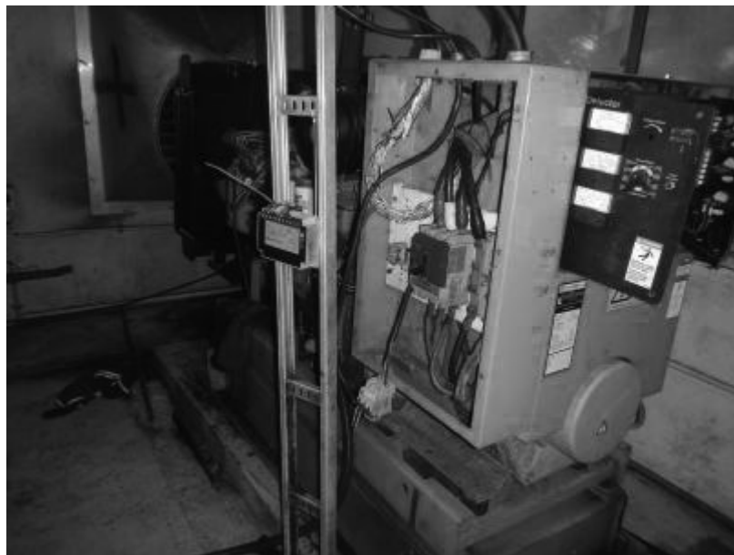
Figure 102: One working generator
