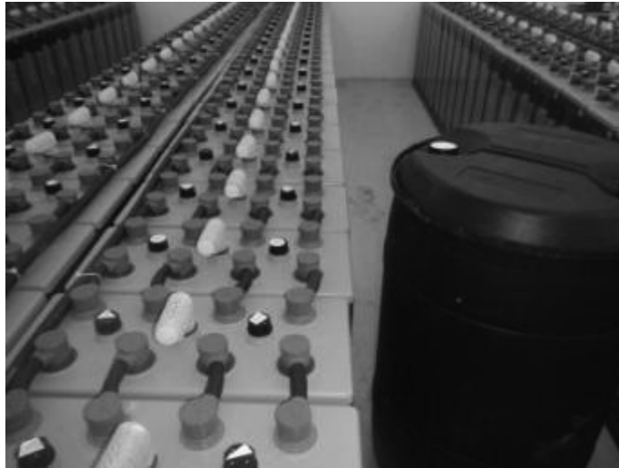
Figure 100: Drum of battery acid obstructing row
