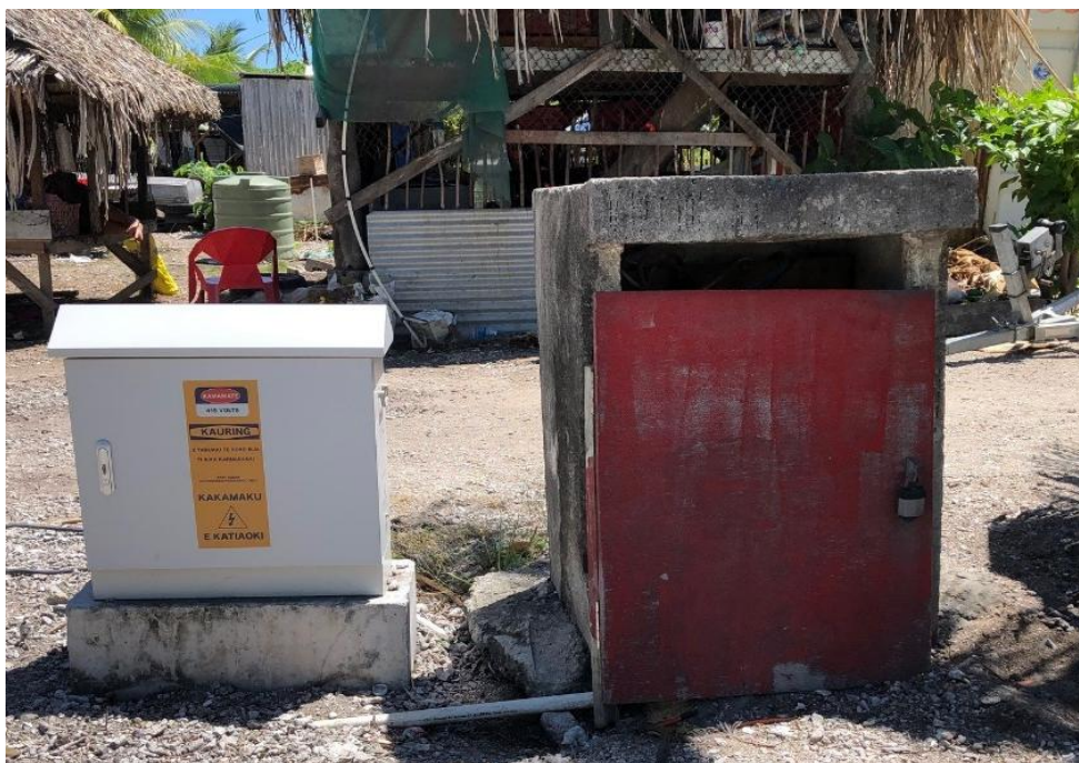
Figure 4: Roadside power boxes (Photo credit: Apisake Soakai)
