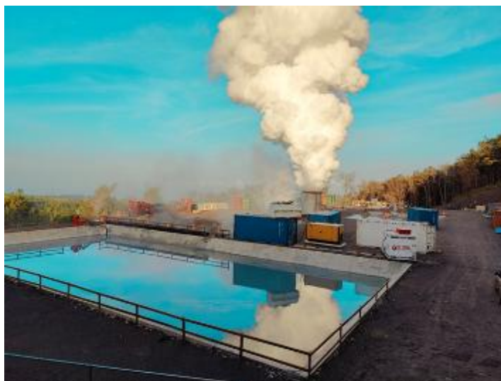
Flow testing a geothermal well in Dominica. Credit: JRG Energy
