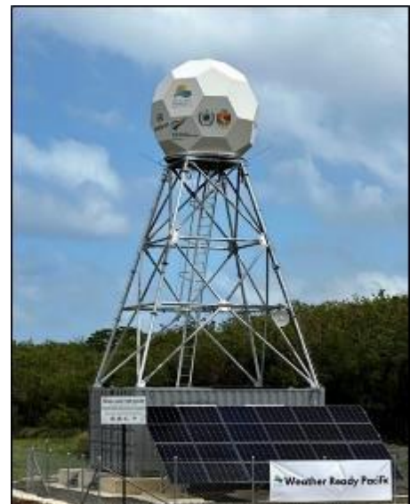
Weather radar at Fua'amotu International Airport. Credit: NZ MetService
